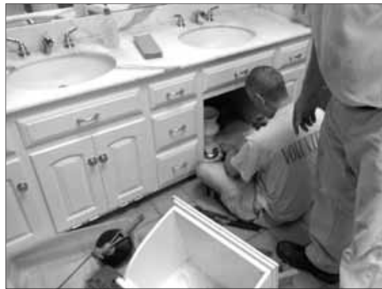
Don Kremer, a member of St. Joseph Church in Conway, repairs a bathroom sink at St. Andrew Church in Danville June 3. Eight men from the Conway parish partnered with the Danville parish for a one-day mission experience.
